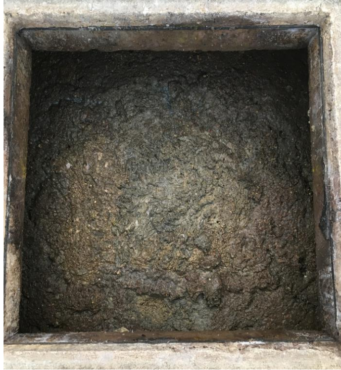
Figure A2: Scum Accumulation in Settler 1A
